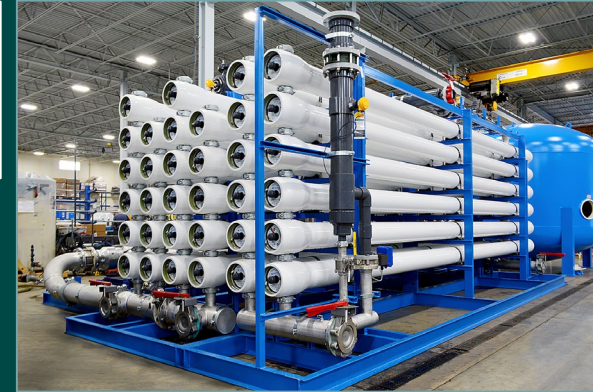
Nanofiltration (NF) and Reverse Osmosis (RO)
